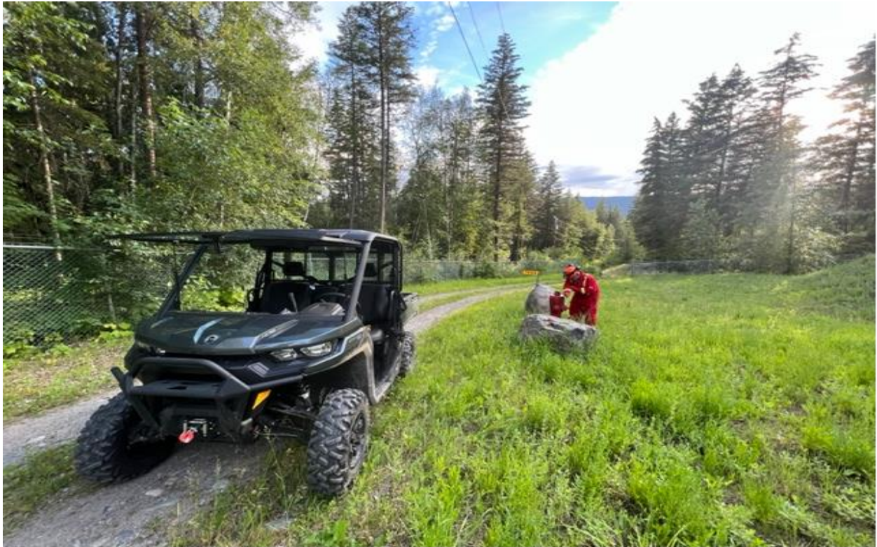
Ron Lampreau Sr, servicing and testing a fire hydrant in the community.
